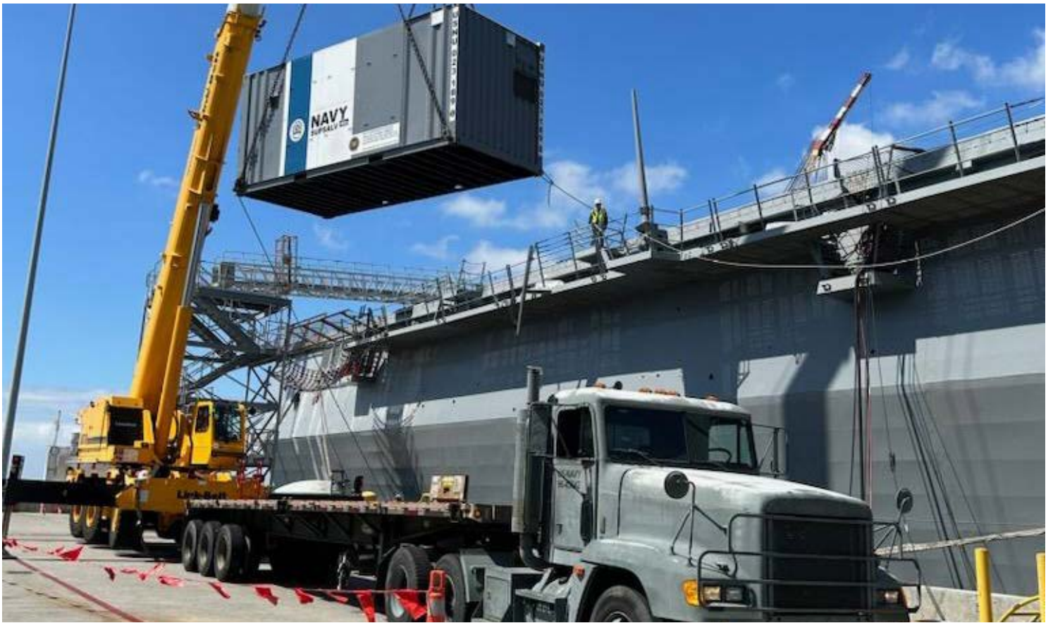
A container with an ADDiTEC ElemX liquid metal 3D printer is transferred aboard the amphibious landing dock USS San Diego (LPD 22) at Naval Base San Diego. Installation of the ElemX by NPS's Consortium for Advanced Manufacturing Research and Education (CAMRE) allows for further testing and evaluation of 3D printing capabilities in an at-sea environment. (US Navy photo.)
