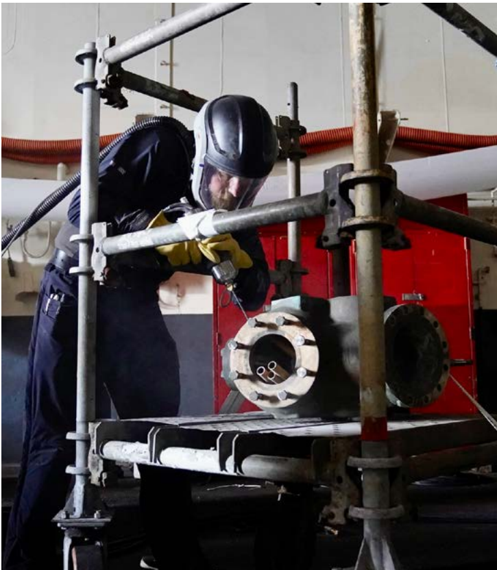
A contractor with industry participant Titomic demonstrates how to use plasma cold spray to fill in a crack on a damaged piece of equipment aboard the USS Tarawa during the REPTX Salv-Ex event in May at PHNSY. (US Navy photo by Claudia LaMantia.)
