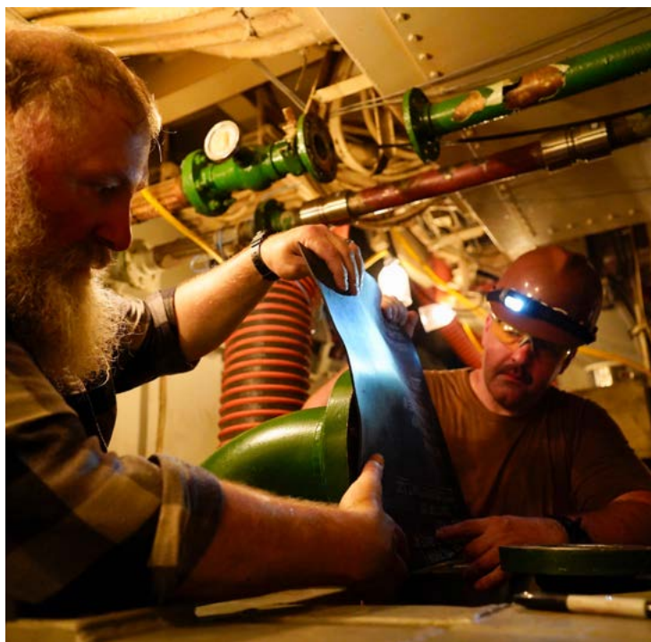
A staff repair technician (left) and a Sailor (right) work on making a rubber gasket aboard the USS Tarawa, a decommissioned ship, during the REPTX Salv-Ex event in May at PHNSY. (US Navy photo by Claudia LaMantia.)
