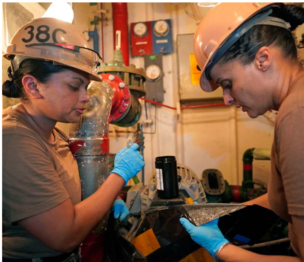
Two Sailors prepare to repair a damaged pipe aboard the decommissioned amphibious assault ship USS Tarawa at PHNSY during the REPTX Salv-Ex event, held May 20-31, 2024. (US Navy photo by Claudia LaMantia.)
