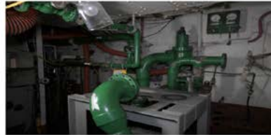
Ex-USS Tarawa engine room
