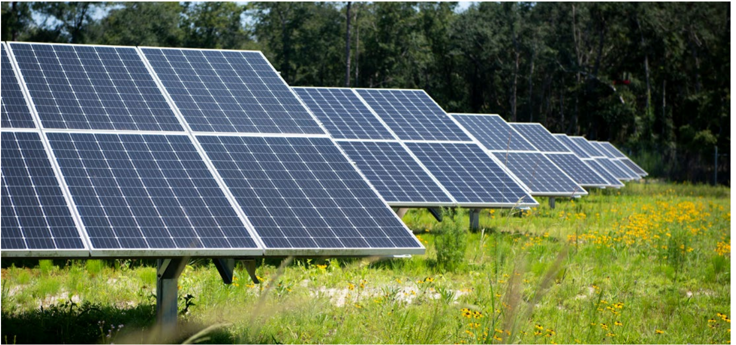
Moody Air Force Base in Georgia had an array of solar panels installed on base during an energy infrastructure project designed to save on energy costs. (US Air Force photo by Airman 1st Class Megan Estrada.)
